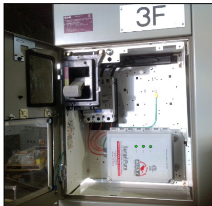
Mach 4 inside 800 amp MCC. Made to fit in switch gear
