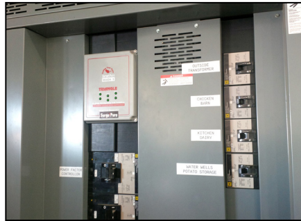
Mach 5 primary level protection. 2000 amp service entrance
