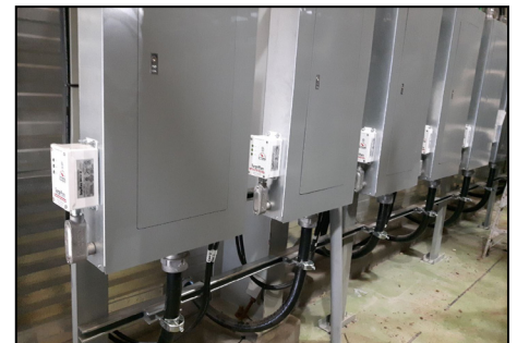
Mach 2 SPDs protecting Canada's Largest Bitcoin operation
